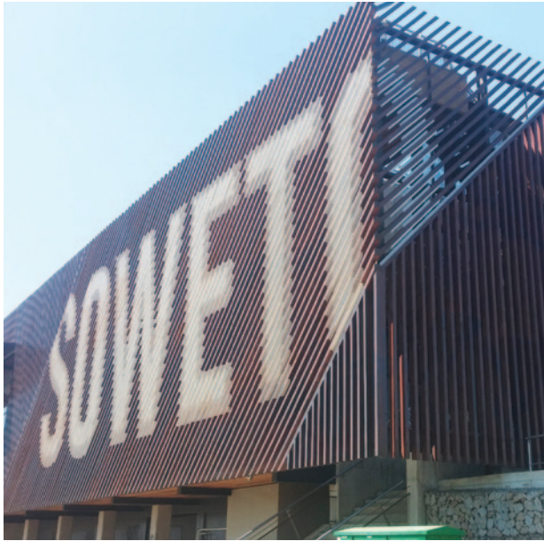
The Nike Soweto Soccer Academy was designed to include 63 x 63 laminated Saligna beams as cladding, highlighting not only the structural integrity of the product, but its bold aesthetic value. Timber supplied by RSB and installed by JB Roofing. Image by RSB.
